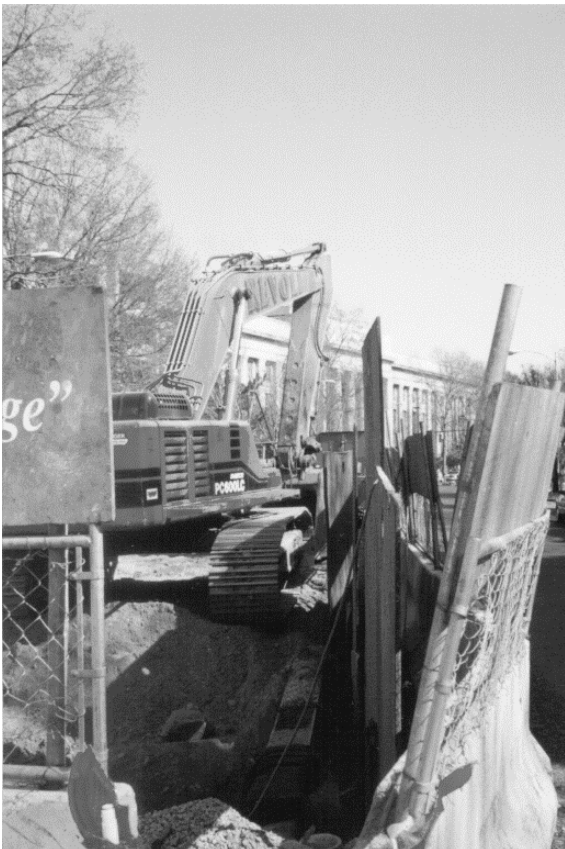
Figure 1 Separating Storm Sewers from Regular Sewers on Massachusetts Avenue, Cambridge, MA In Cambridge and Boston, as in many cities with 19 th century sewer systems, when heavy rains over-taxed the system’s capacity to handle the combined mixture of sanitary waste and rain water, the noisome excess poured was diverted directly into the nearby rivers or the ocean. As part of various projects aimed at cleaning up the Charles River and Boston Harbor, the two cities worked to develop separate systems for storm water, so that only rain water would be discharged into the waterways.
